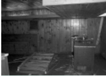
The Chapter Room has been renovated with new lighting and ventilation and removal of the old cooler system. This should alleviate any dampness on the ground floor.
