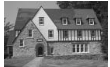
The complete exterior of the house was painted this summer. The wood is in great shape, but the chimneys and roof will need attention in the near future.
